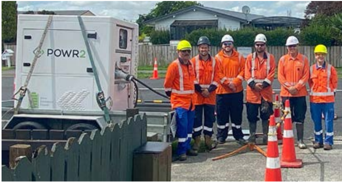
Members of the Powerco, Generator Rental Services and Northpower team with the BESS at Ngātea Early Learning Centre.
