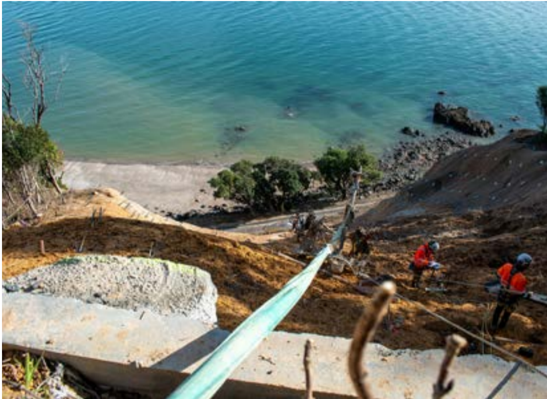
The ground drops away into the large slip above SH25 less than two metres from the house. Photo: ALICE PARMINTER
